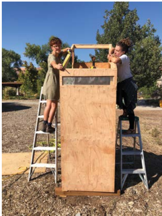
Community Rebuilds interns Eddie Lovell and Eilise Gancarz-Davies preparing to install the roof of the dehydrator
